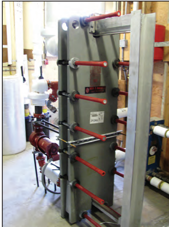
Figure 13 - New Heat Exchanger
