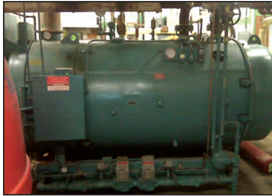
Figure 5 - Old Cleaver Brooks Boiler
