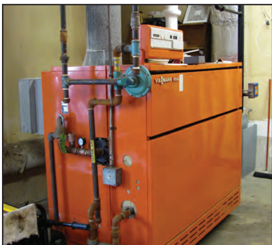
Figure 8 - Viessman Peaking Boiler
