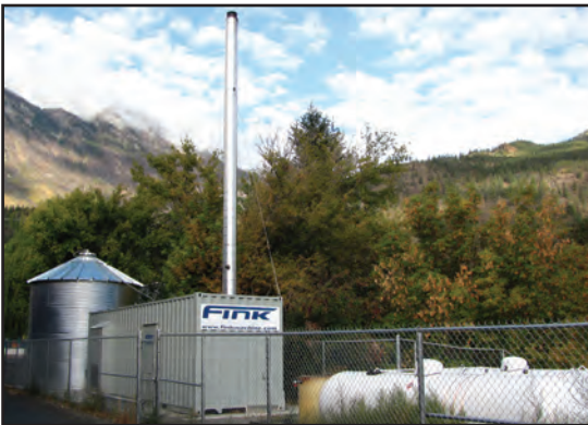
Figure 3 - New Pellet Boiler System
