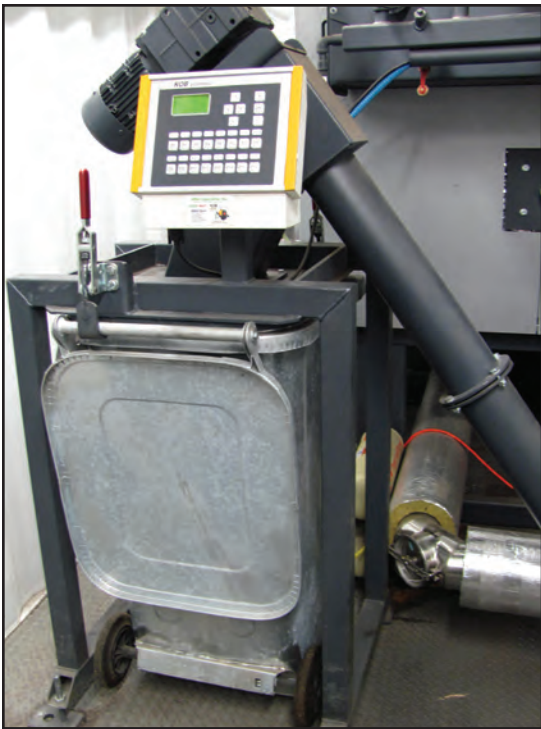
Figure 12 - Ash Collection Bin
