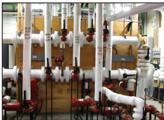
Figure 6 - New Heat Distribution Pumps
