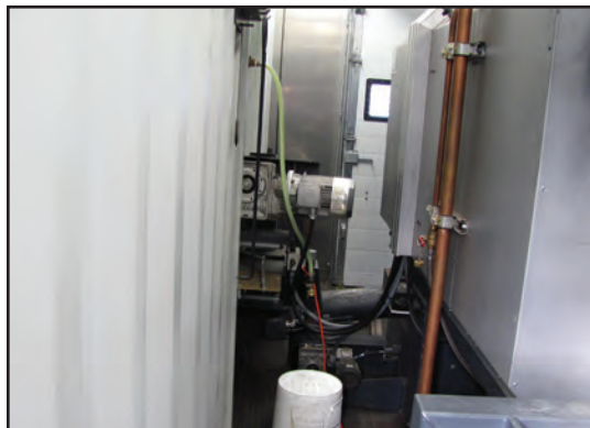
Figure 15 - Pellet Feed System Inside Boiler Container
